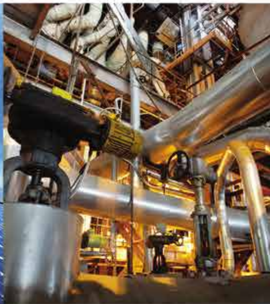
Oil & Gas Plant
