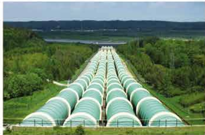
Gigantic water pipes of a power plant
