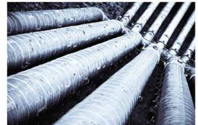
Water pipeline to Hydro-Electric power station
