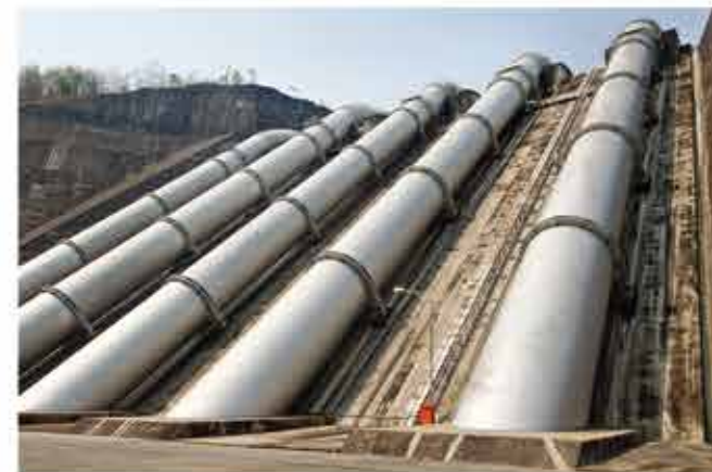
Water pipeline to Hydro-Electric power station
